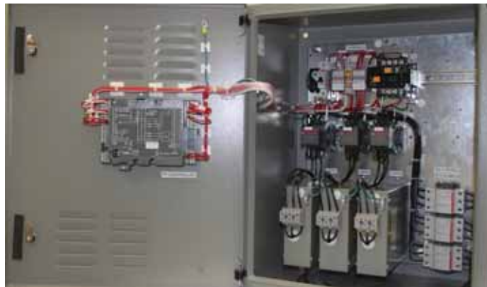
S100 plain cap bank up to 45 kvar with space for incoming splitter or breaker
